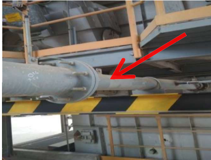
Gambar.3a Saluran Pipa Calsiner Burner
